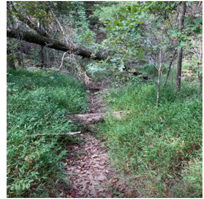
Paved ditch blocked by vegetation
